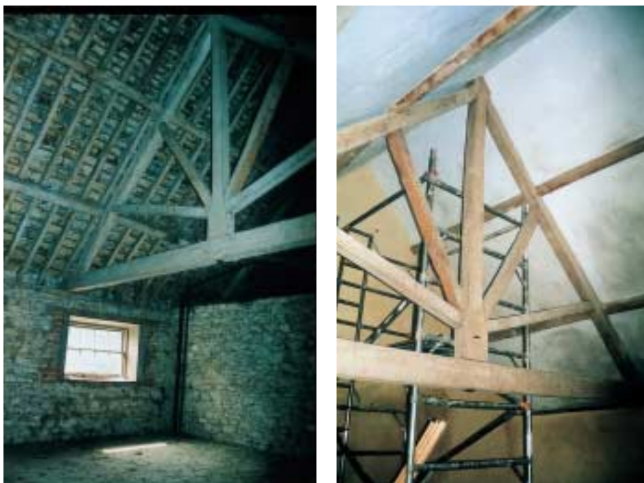
Figure 12 An attic being converted for use as a habitable room where the requirement was not to strip the stone slates. Traditional torching prevents ingress of driven rain, and protection and thermal improvement is provided by: torching a lightweight permeable building paper to underside of rafters, natural wool insulation, cellulose/jute batts, wood fibre boards and a lightweight mineral wool insulation board (or reed board) coated with lime plaster and subsequently limewashed. (Photographs courtesy of Richard Oxley, Oxley Conservation, © Richard Oxley)
